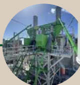
New batching plant Hal Far
